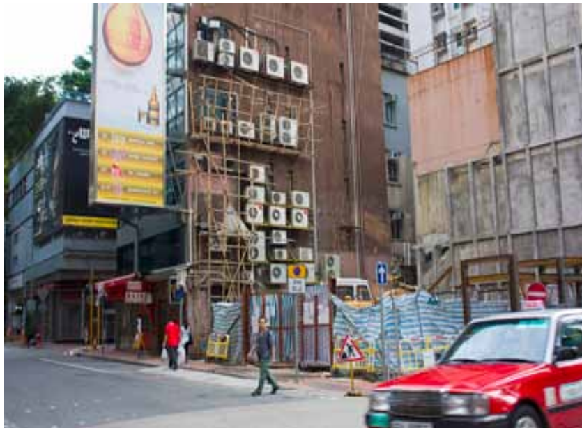
Figure 20: Barnacles of air conditioning units in Hong Kong
